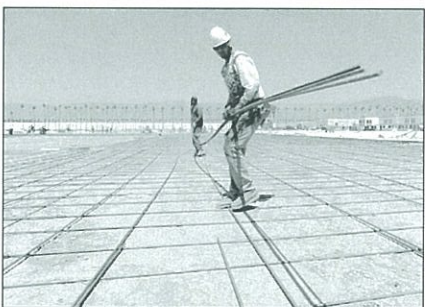
ERIC TOM/Staff Photographer Steven Gomez, left, and Jaime Barba Vargas lay out rebar for a 616,000-square-foot industrial building in northwest Redlands on Friday.
