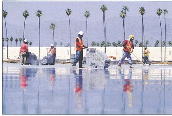
A section of the concrete floor for a 616,000-square-foot industrial building in northwest Redlands is worked on Friday. The building is expected to be finished by the beginning of September, said Dave Harper, Millie and Severson Incorporated superintendent.
